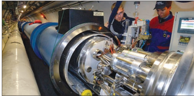
Left: The final superconducting magnet for the LHC begins its descent into the accelerator tunnel. Right: Brazers work on the last octant between Points 1 and 2.
